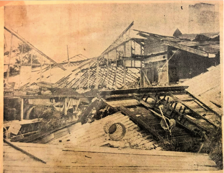
THE COLONIAL GREENHOUSES on Shore Road are shown after a windstorm whirled through Somers Point and the southern tip of Linwood yesterday. This greenhouse collapsed and windows of other greenhouses owned by Theodore Meskers were blown out. Meskers and his brother, Herman, said they had no insurance on the nursery section of the property.
